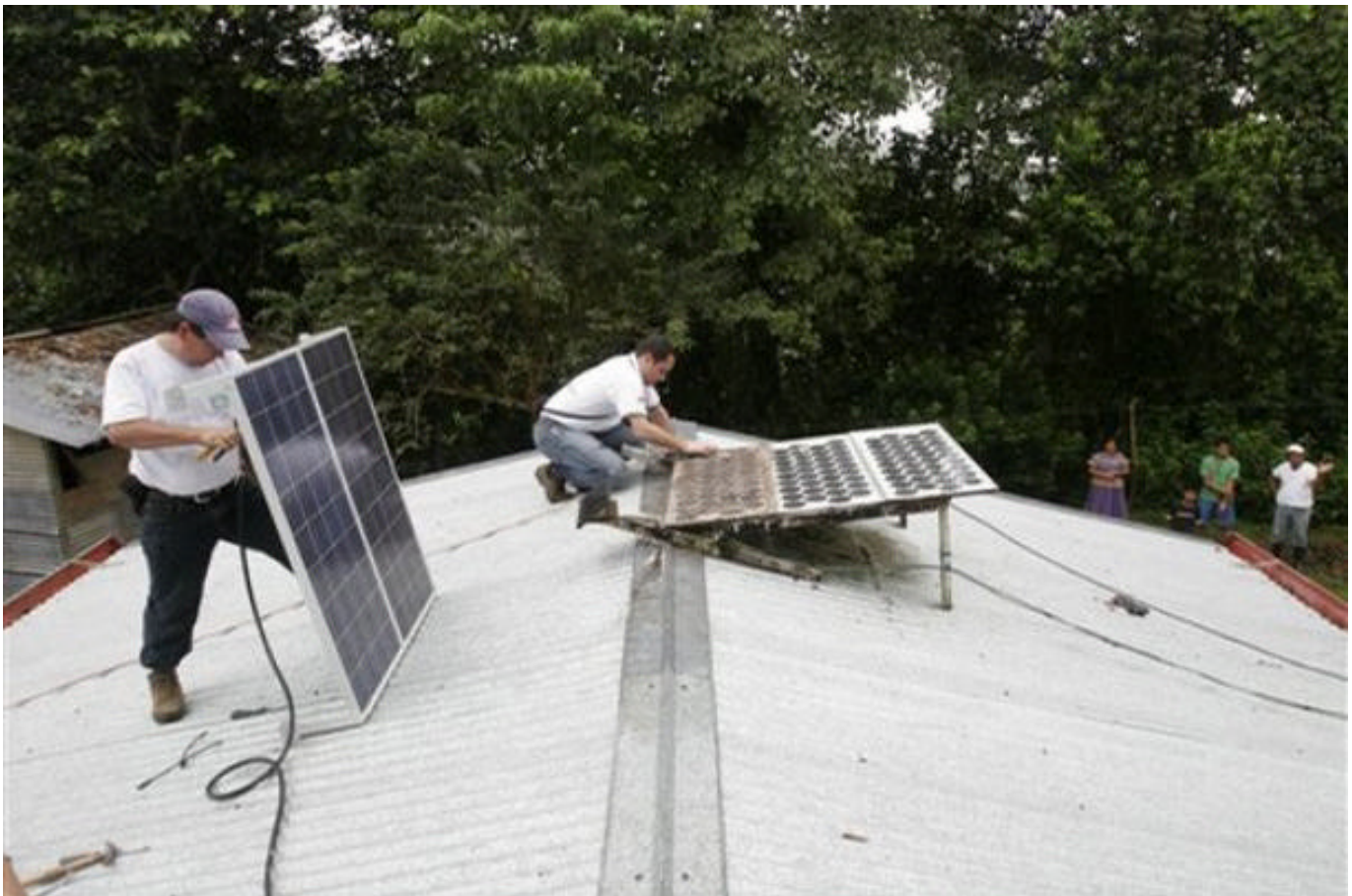
Workers install a new solar panel, left, to power a refrigerator and clean algae from an older solar panel, right, in the village of Alto Conte, at the Brunca Indigenous Reservation in southern Costa Rica, Thursday, Nov. 8, 2007. AP photo by Kent Gilbert.
